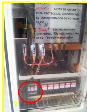
2. Valvetrab in A compartment 2. Valvetrab en compartimento A
